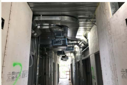
2 nd Flr. MEP infrastructure
